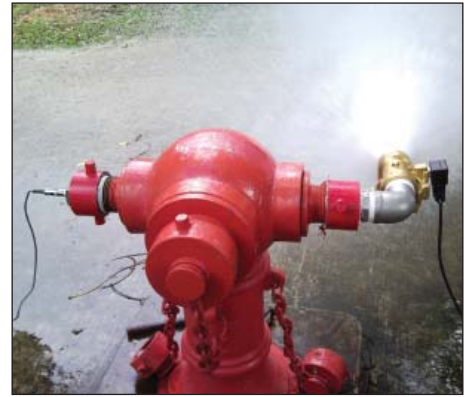
During leak-off experiments artificial bursts and leaks were generated by rapidly opening solenoid valves connected to fire hydrants.
